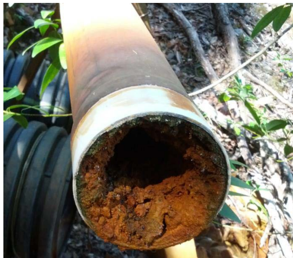
Figure 5. Precipitate clogging a test pipe in the Lower Corona drain tunnel outlet.
